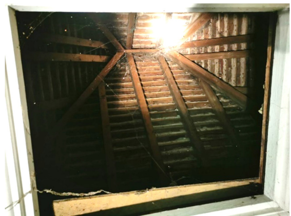
Photograph 4. View of loft space structure with no lining.
