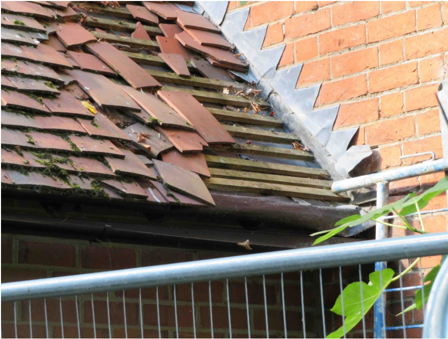
Plate 16 – Potential bat access points into lodge.
