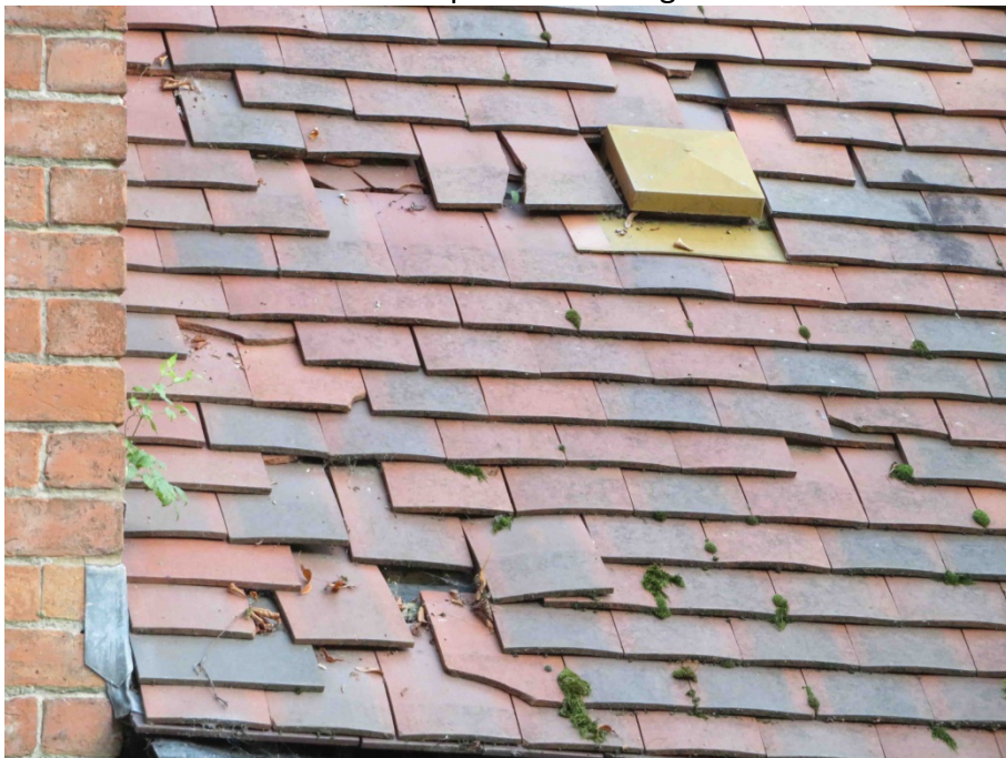
Plate 15 – Potential bat access points into lodge.
