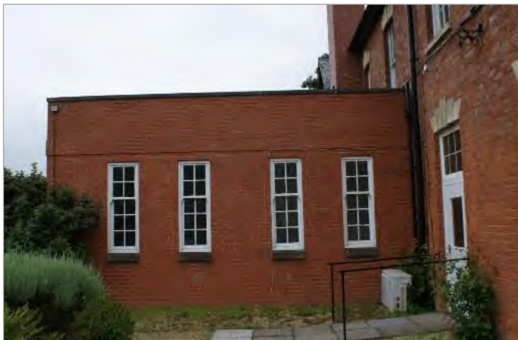
Plate 19. Poorly detailed east elevation of southern extension.
