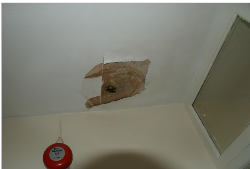
Plate 18. Minor cosmetic damage from water ingress.
