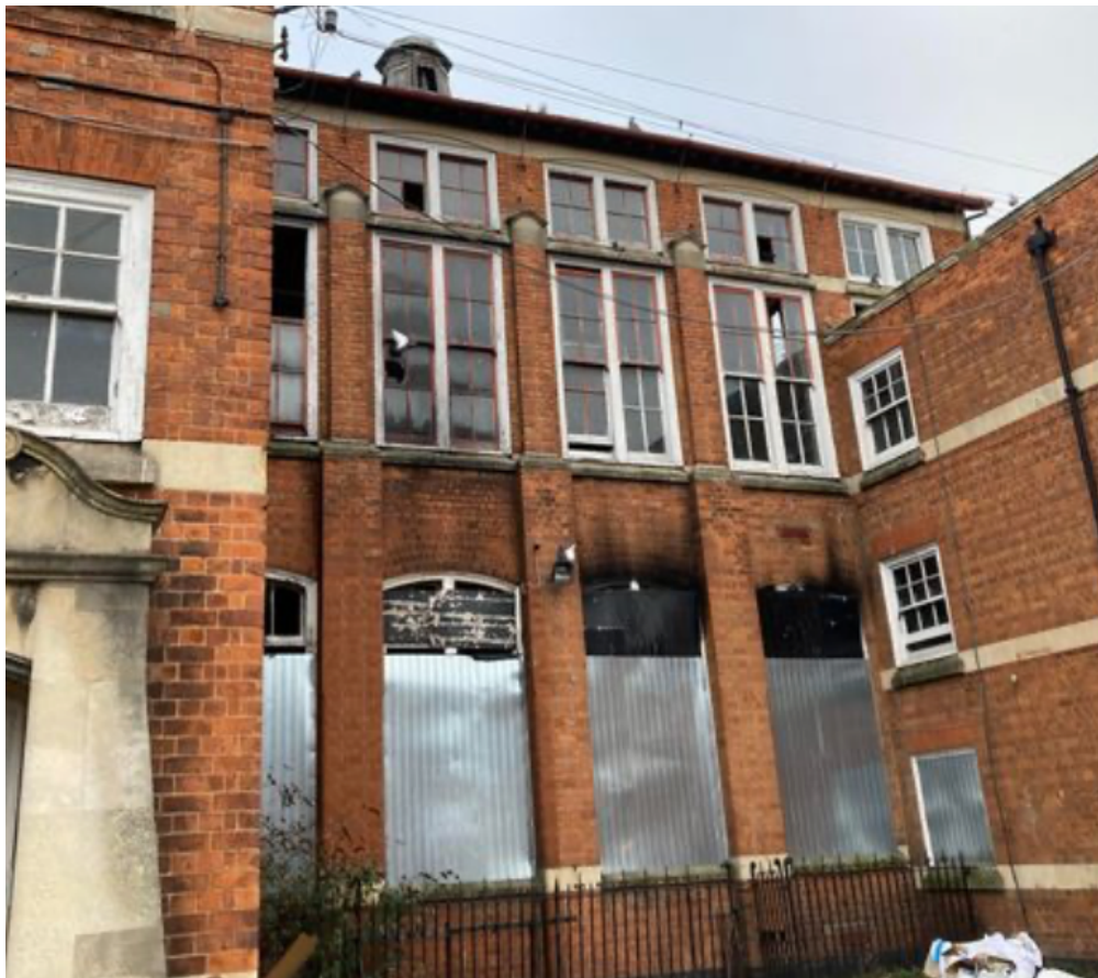
Photographs showing fire/smoke damage from January 2022 (Source – Gloucestershire Live)
