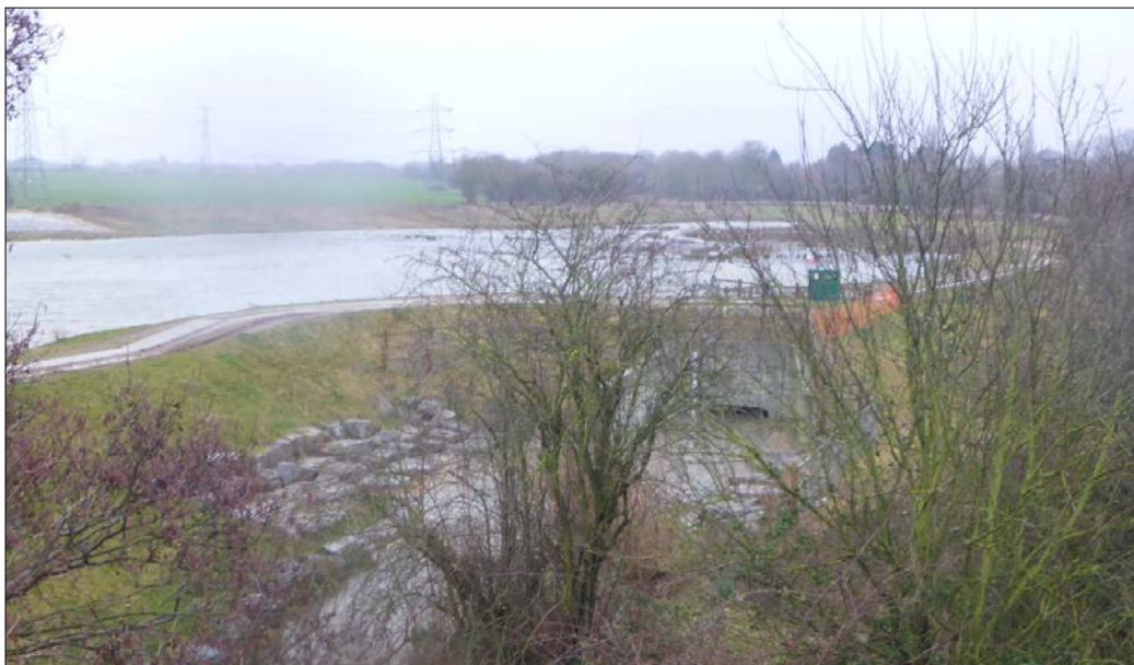
Figure 1-3 Photograph of Horsbere Brook FAS partially full following recent wet weather (February 2014)
