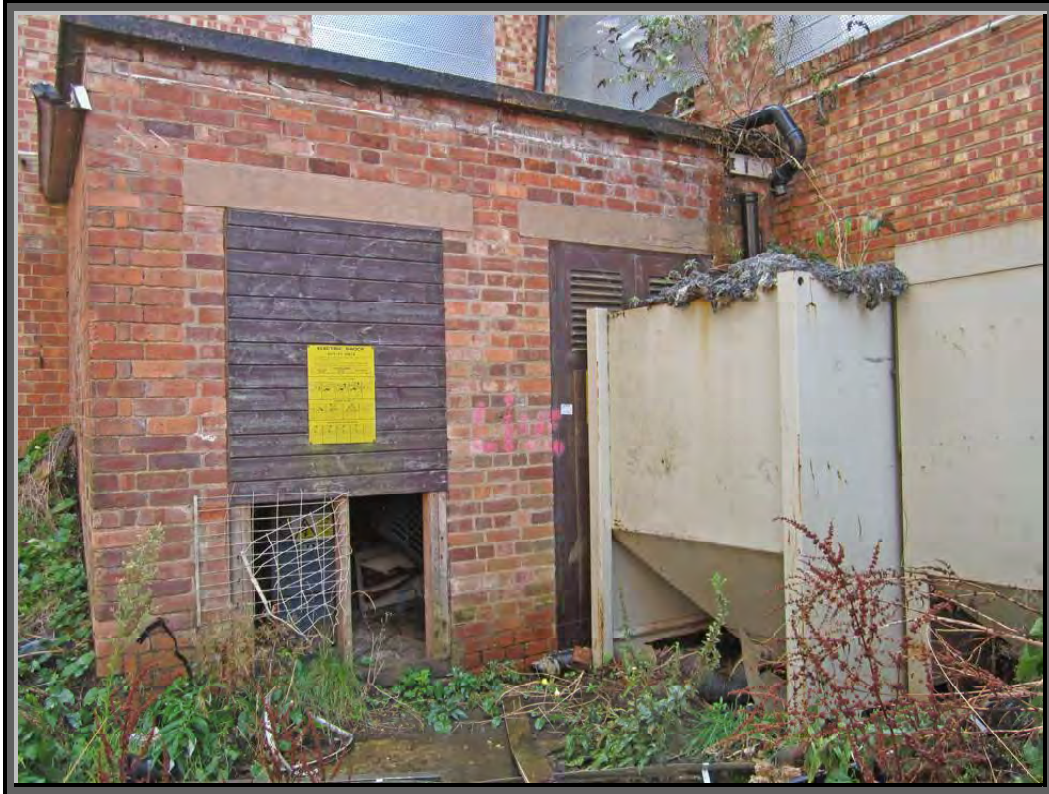
Photograph P7: showing redundant electricity sub-station
