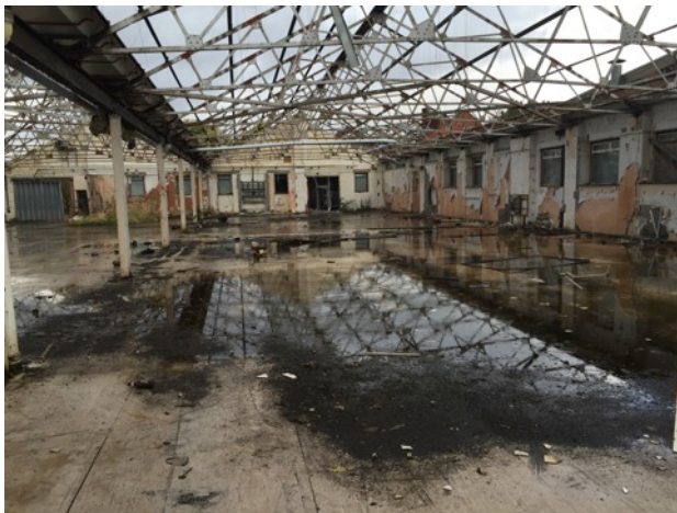
Photograph 8: Main section of Building 1 with missing roof.
