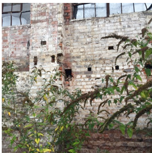
Photograph 18: View of holes in the southeast wall of former Building 5.
