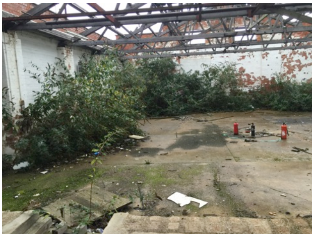
Photograph 10: End section of Building 1 with missing roof.
