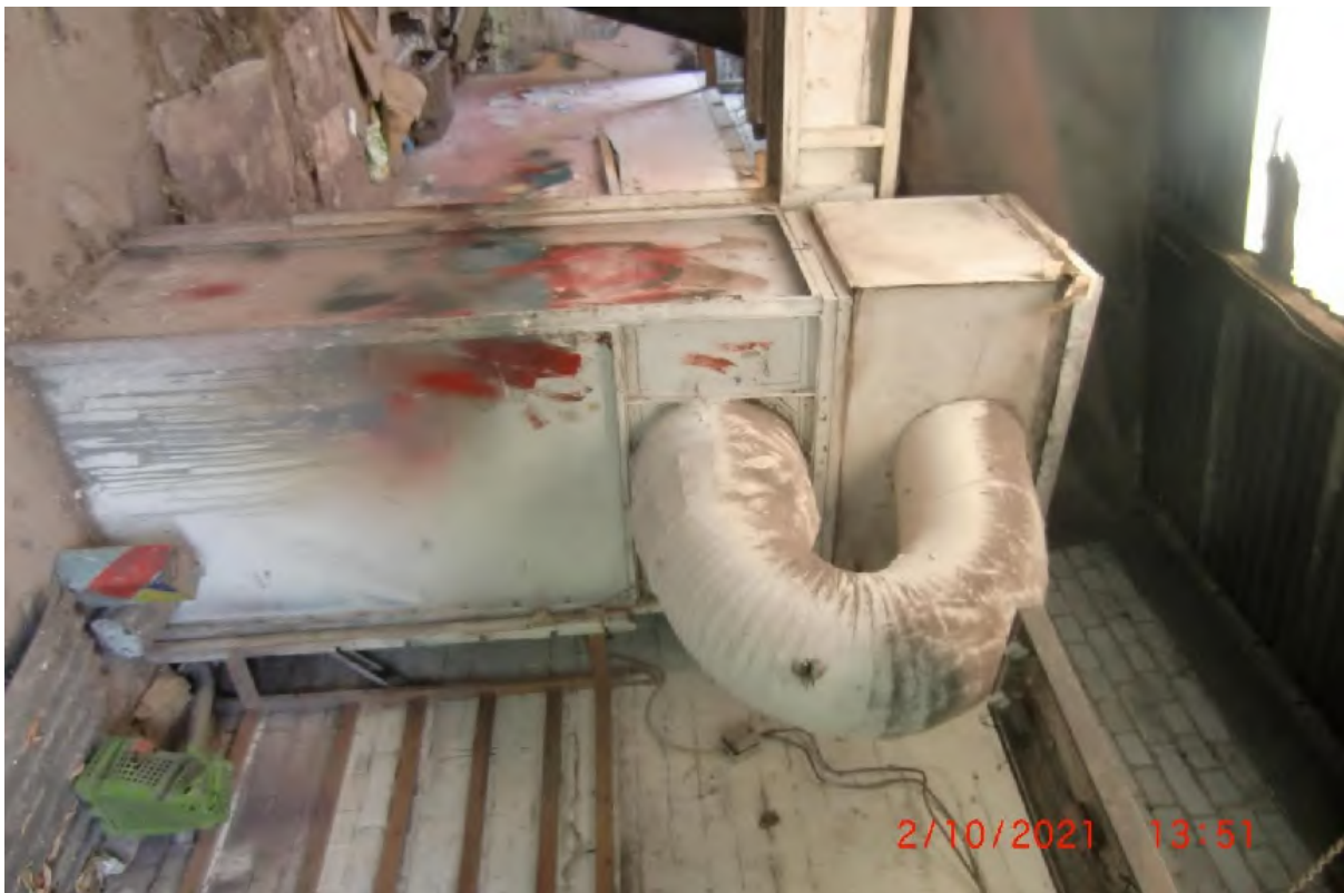
Extractor unit in spray shop
