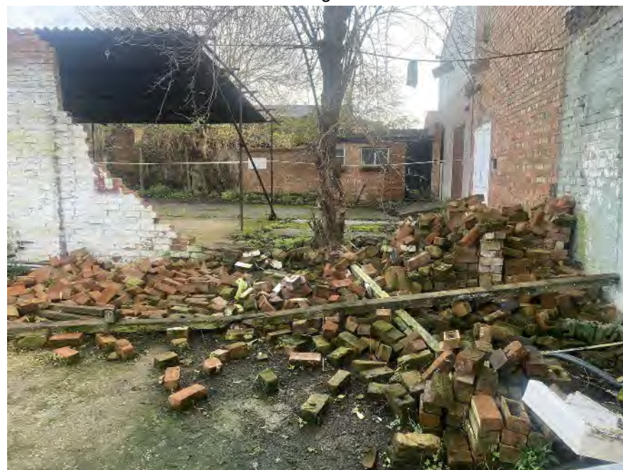
Collapsed Boundary Wall
