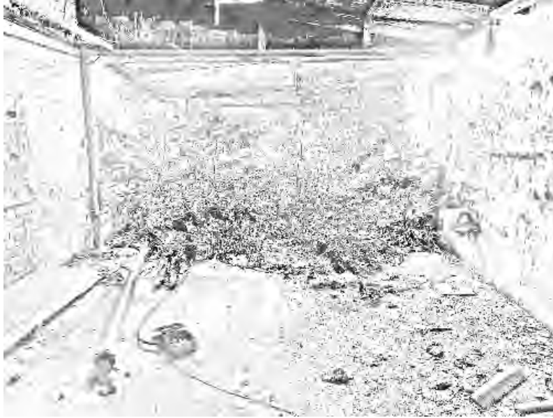
Existing Over grown bush growing throughout the building
